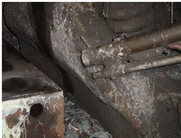
Figure 13. Open tube nozzles directed toward hammer block. Photo by NIOSH.
