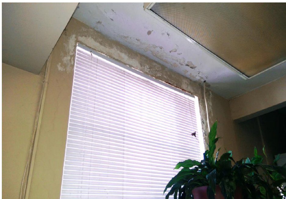
Figure 8. Water intrusion near an office window, September 2014.
