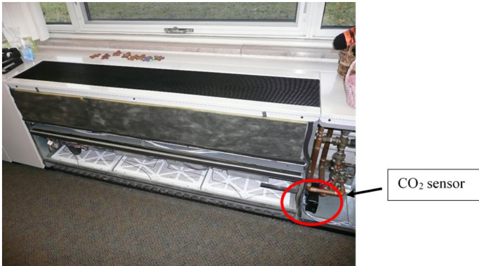
Figure A8. Interior of a typical classroom unit ventilator. Photo by NIOSH.
