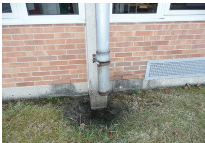
Figure A6. Broken and disconnected exterior roof drain outside classroom. Photo by NIOSH.
