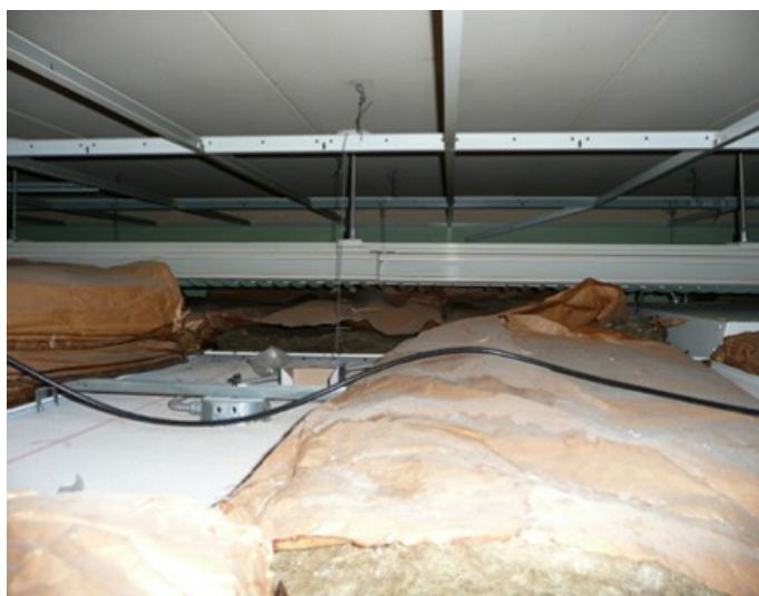
Figure A4. Dusty roll-faced insulation in plenum above classroom. Photo by NIOSH.
