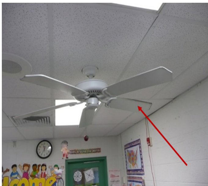
Figure A5. Dusty ceiling fan blades in classroom. Photo by NIOSH.
