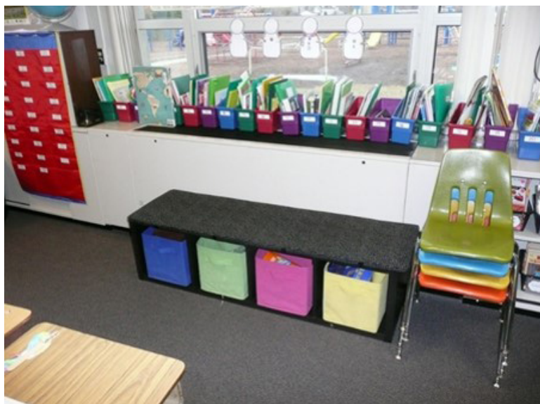
Figure A9. Storage cabinet (on floor) and teaching supplies (on top) blocking air intakes on a classroom unit ventilator. Photo by NIOSH.
