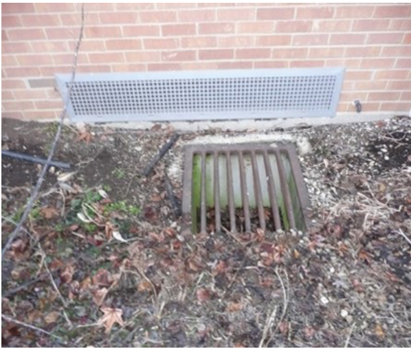
Figure A7. Debris in shallow dry well near outdoor air intake for classroom. Photo by NIOSH.
