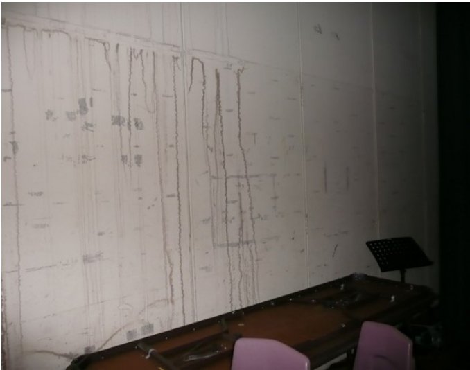
Figure A1. Old water stains on auditorium wall. Photo by NIOSH.
