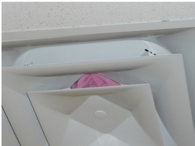
Figure A10. A blocked ceiling mounted diffuser in an office. Photo by NIOSH.
