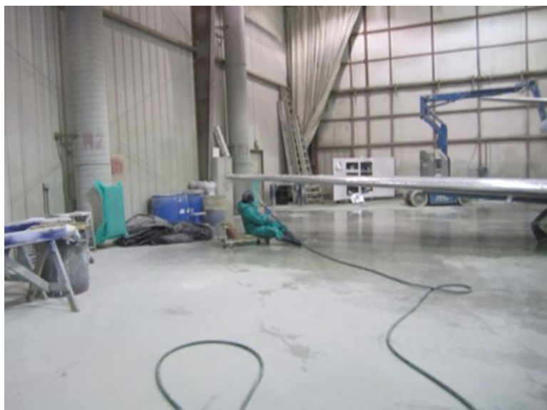
Figure 10. Stripping bay floor level exhaust with paint arresting filters (green filter media covering exhaust hood). Photo by NIOSH.
