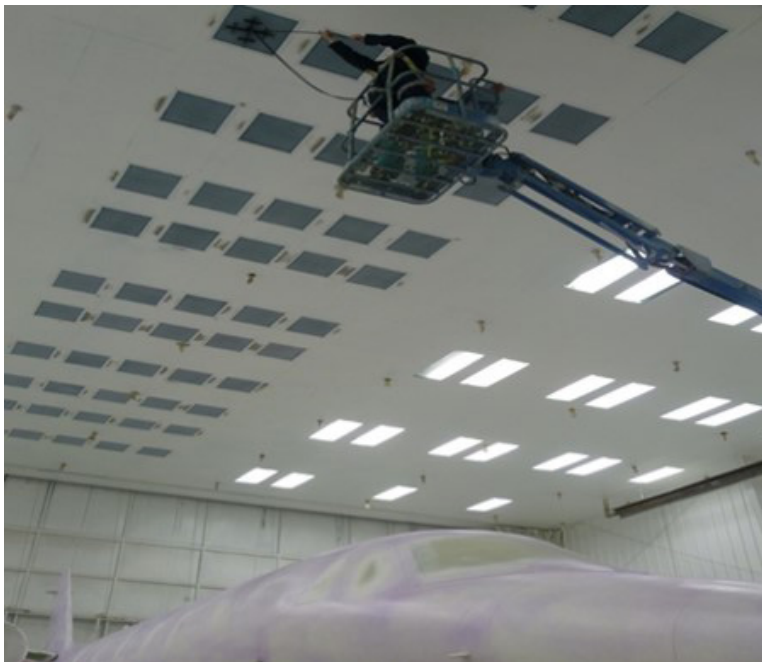
Figure 11. Measuring air velocity and airflow through each of the supply registers in paint bays 1 and 2. Photo by NIOSH.
