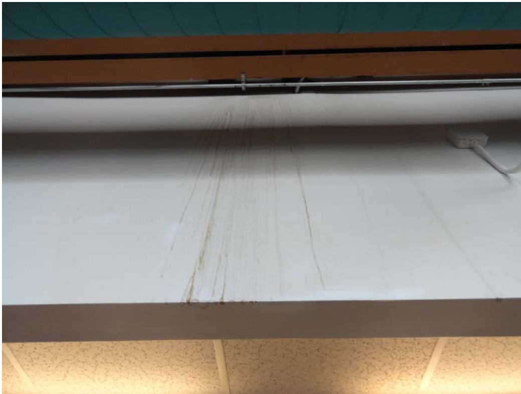
Figure B4. Evidence of recent water damage at an office building on June 1, 2018. Photo by NIOSH.
