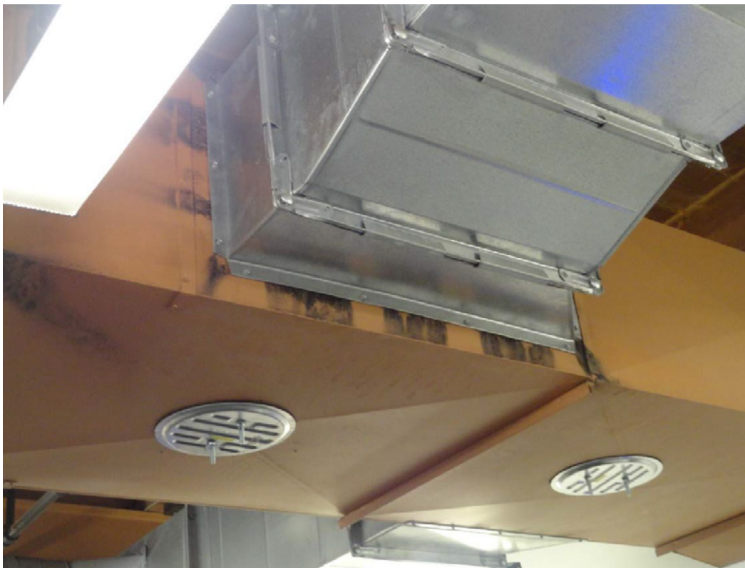
Figure B2. Example of black dust from heating, ventilation, and air-conditioning system at office building on June 1, 2018. Photo by NIOSH.
