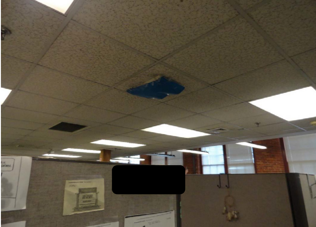
Figure B1. Vent blocked in personal workspace at office building on June 1, 2018. Photo by NIOSH.
