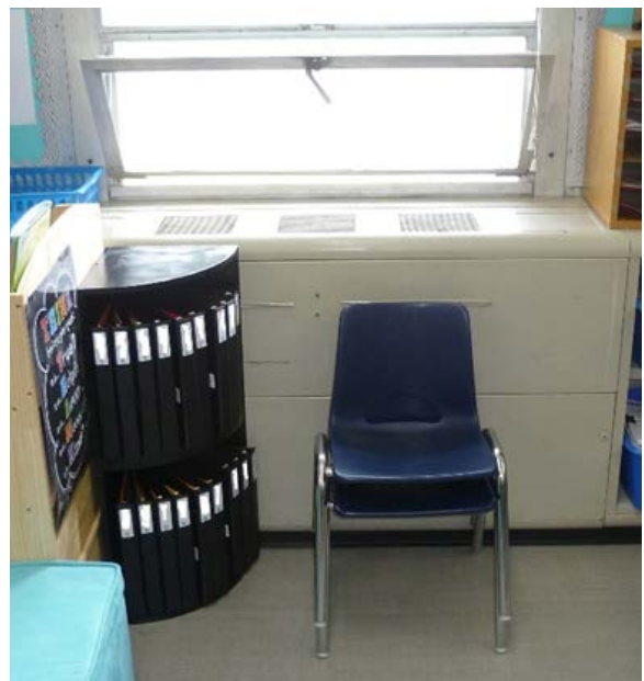
Figure 1. A classroom unit ventilator is partially blocked by furniture and classroom supplies. The window above it is open. Photo by NIOSH.
