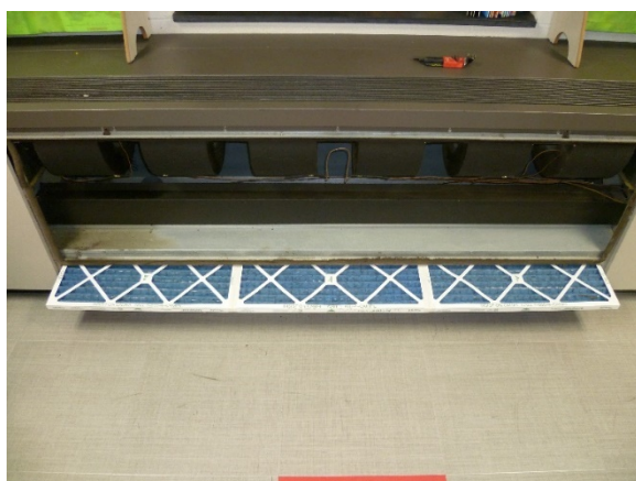
Figure B3. Classroom unit ventilator with access panel removed. Photo by NIOSH.
