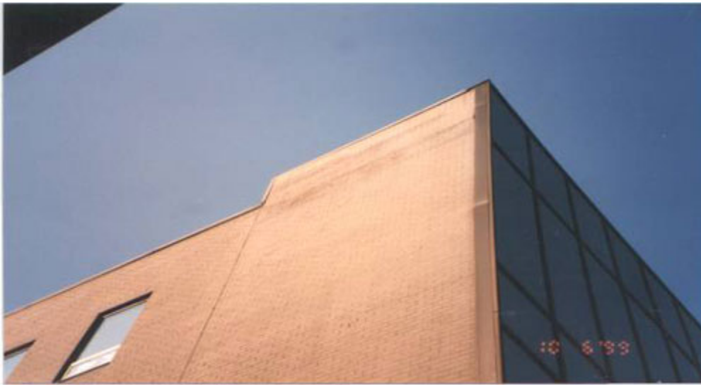
Side of Building Accident Occurred
