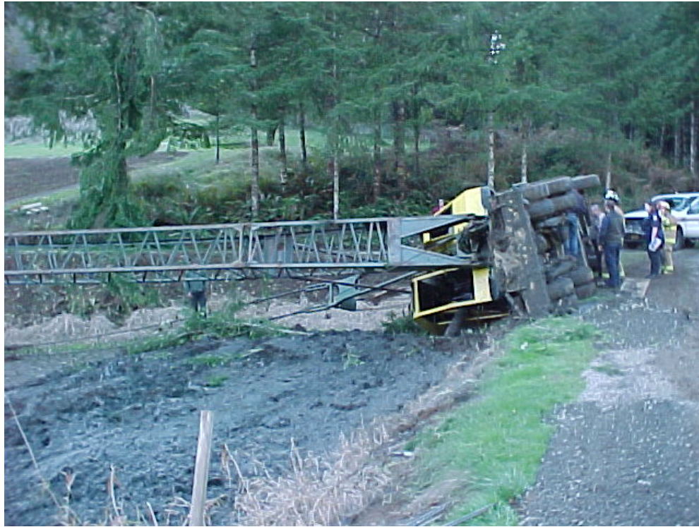
Photo 2. Crane topples over, crushing worker, while dredging dry fish pond. Note: outriggers were not deployed.
