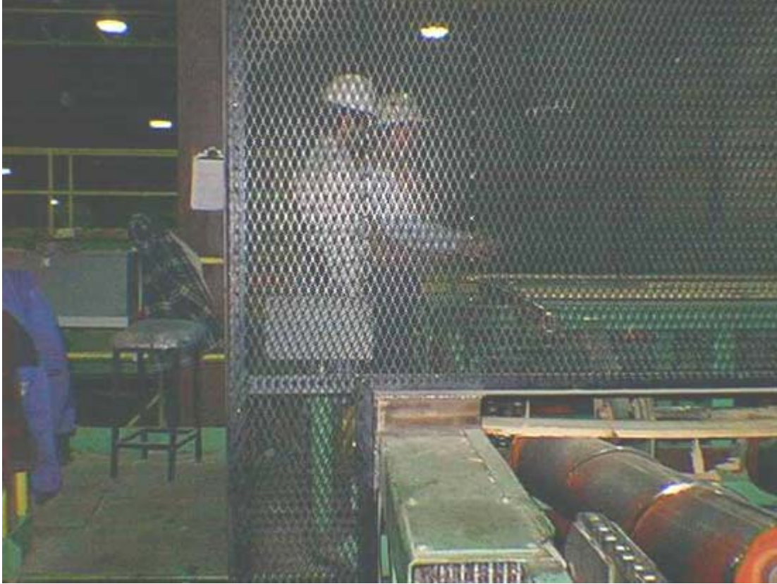
Photo #2. "Unscrambler" operator's station viewed from "trimsaw" operators work station. New Guarding in place.
