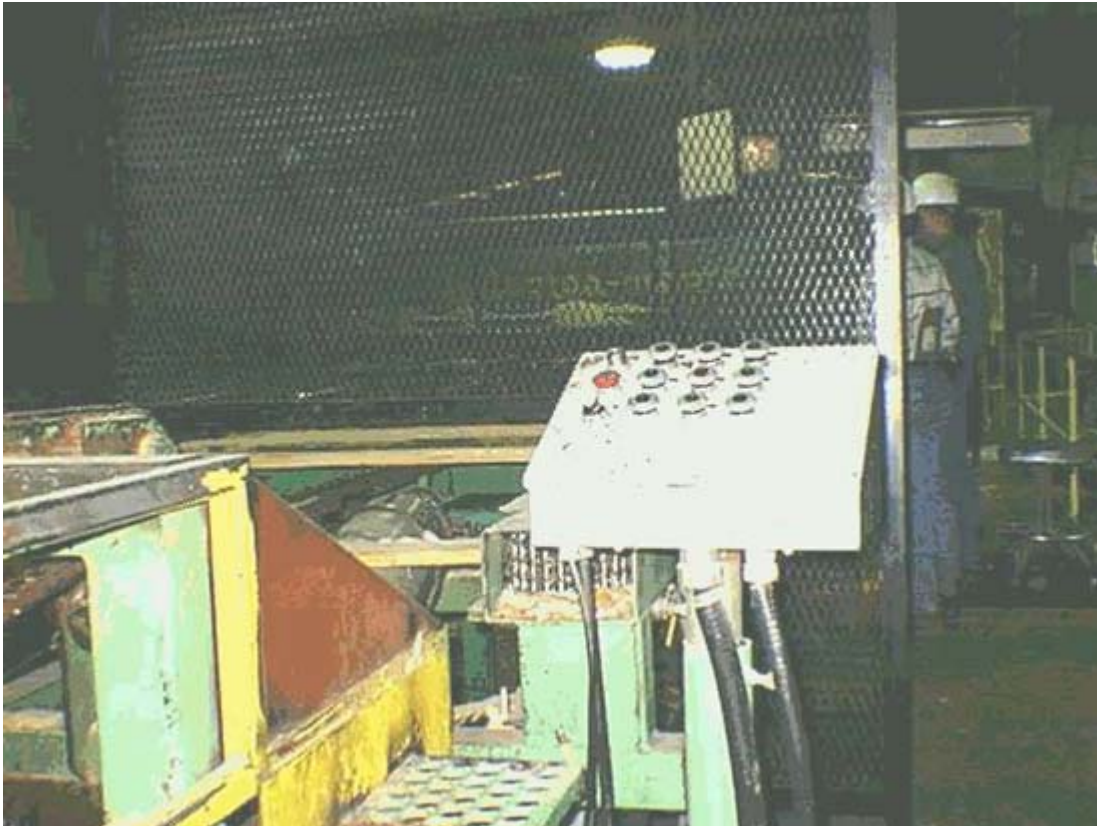
Photo #1. "Unscrambler" operator's workstation - facing "trimsaw" operators work station and trimsaw system. New guarding in place.
