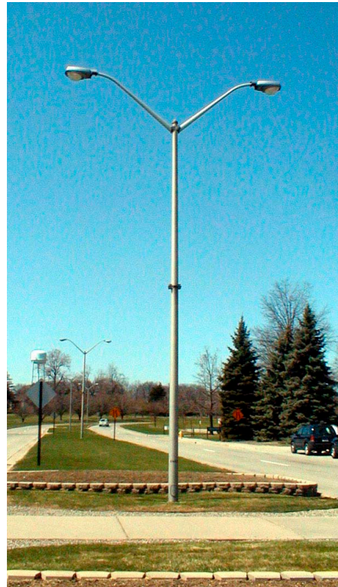
Figure 1 Light pole involved
