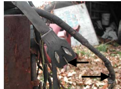
Figure 2-Ground prong loose and damaged insulation
