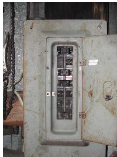
Figure 7. Unlabeled circuit breaker box in shed
