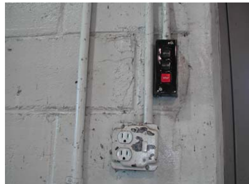
Figure 2. Remote garage door opener by pedestrian door
