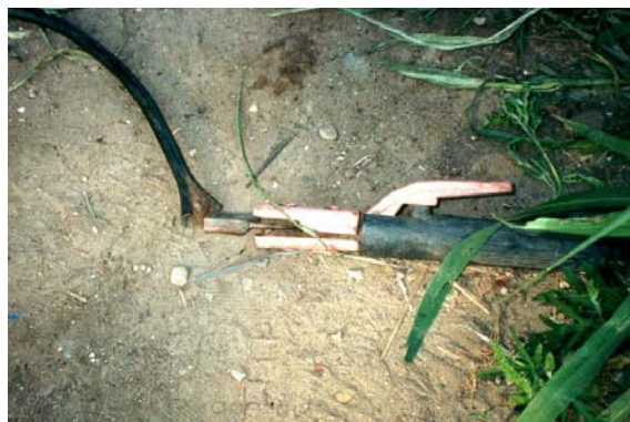
Figure 5. Un-insulated splice on bare ground
