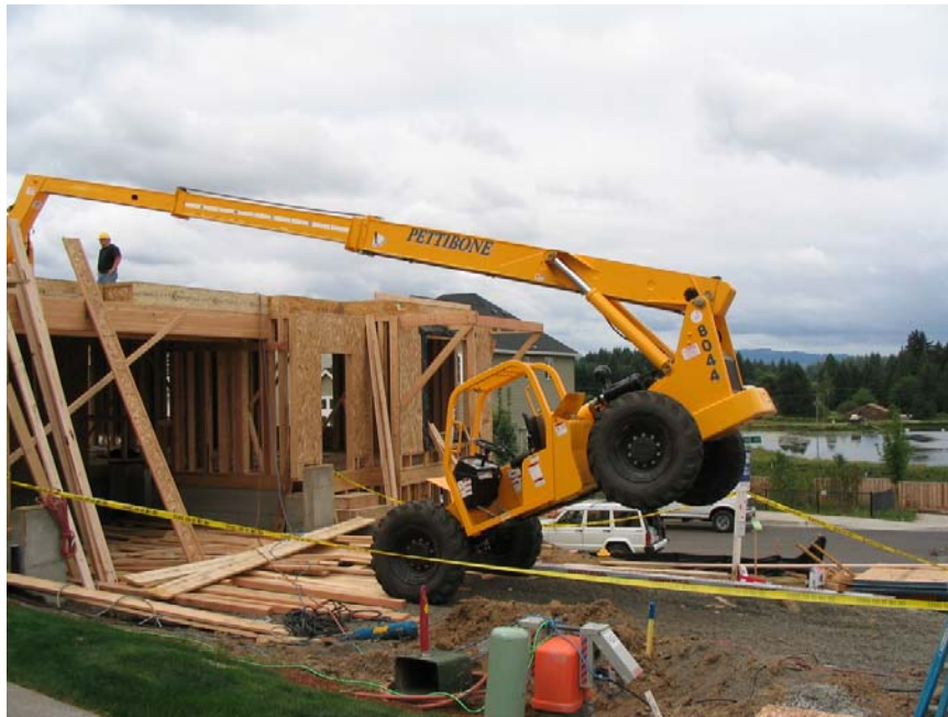
Photo 1. Forklift in position after the load came down. Note board pile in front of the forklift, preventing the forklift from getting closer to the second story.
