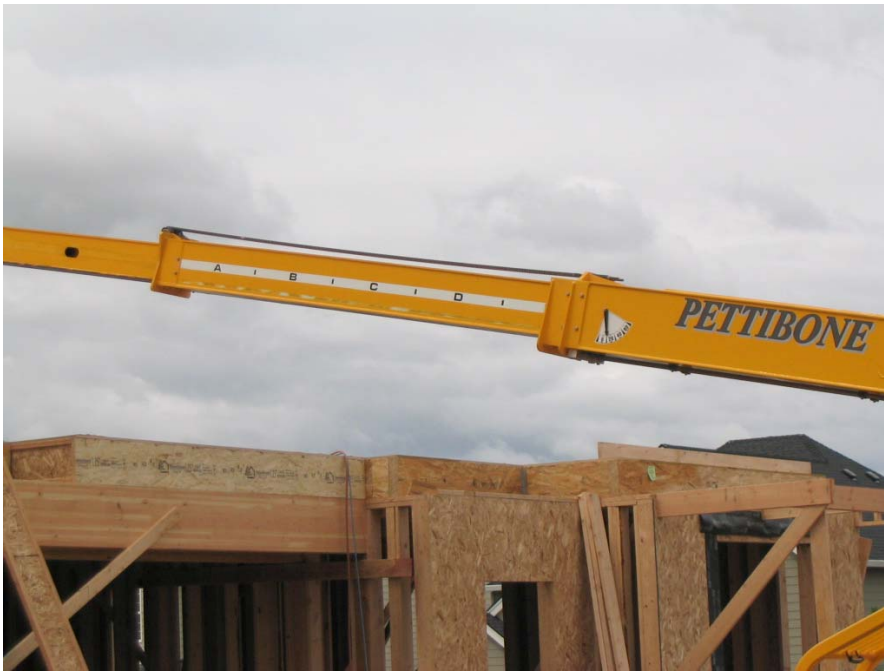
Photo 4. In upended position, the boom is extended between "D" and "E" load rating. Weight of load was calculated to be 3600-3800 lbs. extended ~24ft. The maximum load range at this reach and arc is 2000-3000 lbs.
