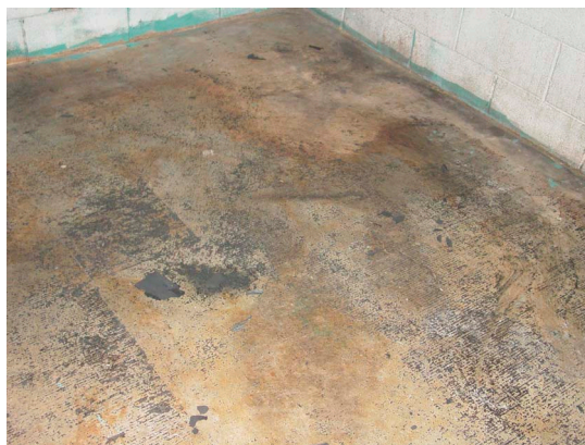
Figure 4. Carpet glue remnants on den concrete floor
