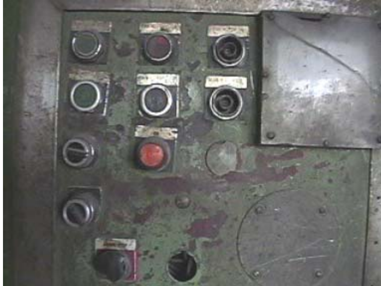
Exhibit #6 View of the machine control panel
