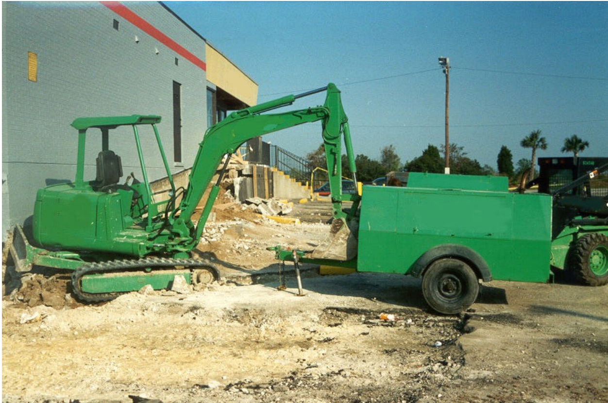
Photo 1. Mini-Excavator. The mini-excavator used in the incident had a 23-inch-wide bucket attached. A bystander was stuck by the bucket and then the bystander and the victim were pushed against an air compressor.
