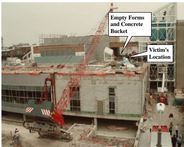
Photo. Crane Tip-Over at Library Expansion Project (Photo courtesy of The Blade/Toledo, Ohio)
