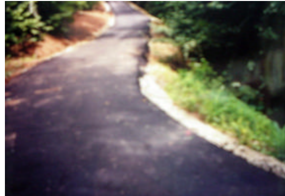
Embankment of Roller Incident
