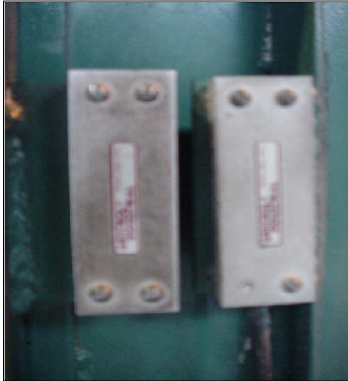
Figure 5. Door safety interlock
