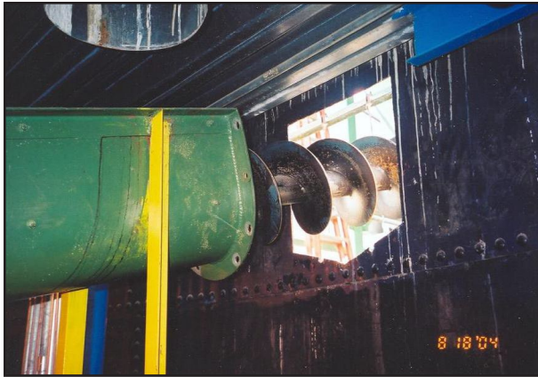
Photo 5. Partially disassembled transfer unloader auger system exiting the silo
