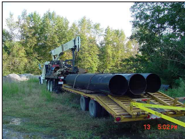
Photo 3. This photo illustrates the sections of pipe on the truck trailer into which the steel augers were to be inserted. [Photograph courtesy of NCOSH].
