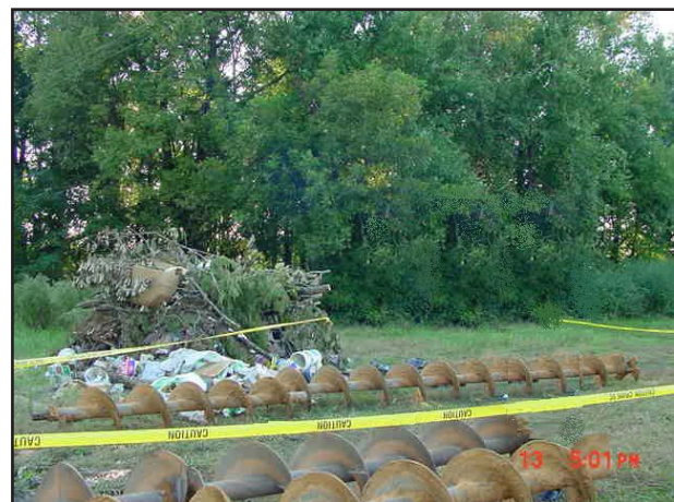
Photo 4. This photo illustrates the steel augers that were being lifted with the truck crane and inserted into sections of steel pipe located on the truck trailer. [Photograph courtesy of NCOSH].
