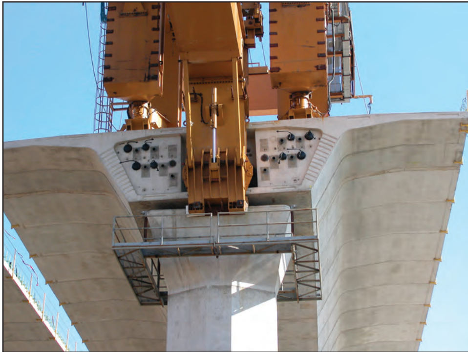
Photo 2. Pre-cast bridge segments in place at end of completed roadbed. The rear legs and underbridge of LG1 are visible at top of photo. Note the horizontal lines on the bottom of the completed bridge which indicate individual precast segments.
