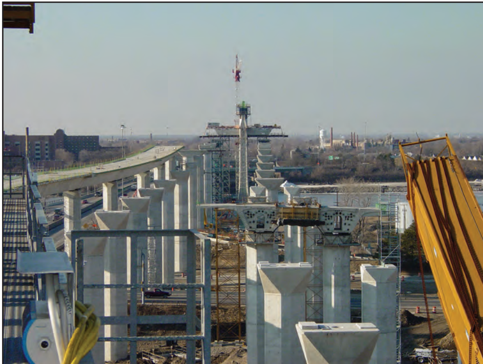
Photo 3. Cast-in-place concrete piers ahead of collapse site. Photo is facing north.
