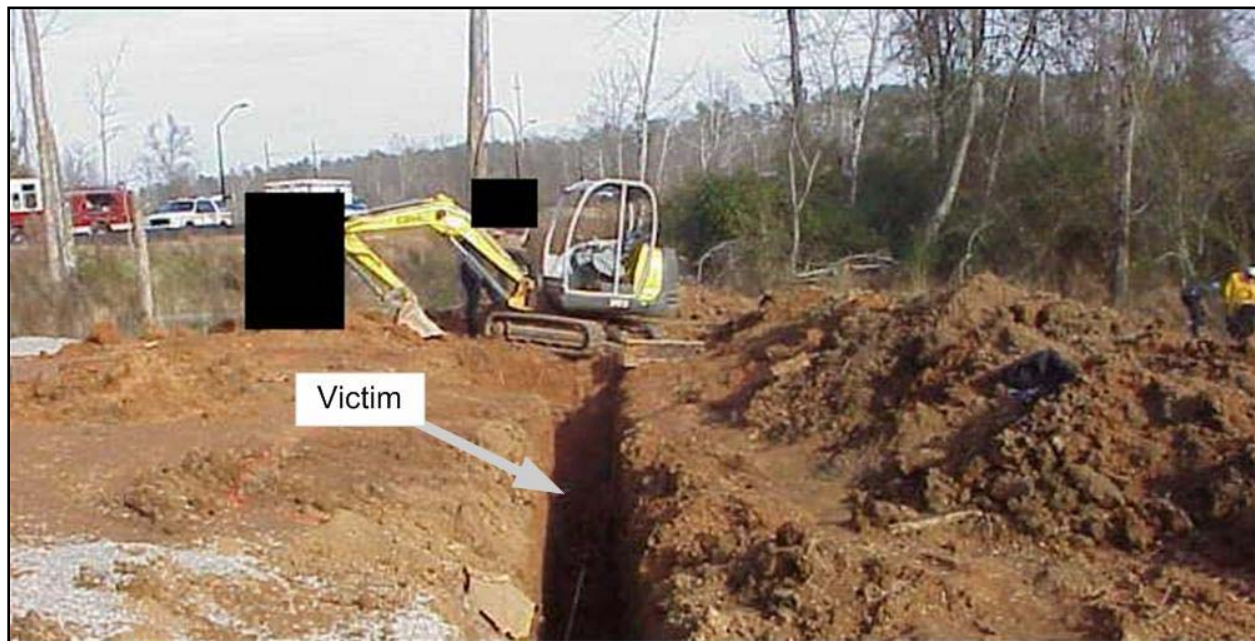
Photo 2. Illustrates the position of the mini-excavator at the time of the incident and the approximate location of the victim.
