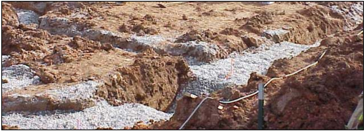
Photo 1. Illustrates the usual depth of the footings and the gravel fill. Photo courtesy of NCOSHA.
