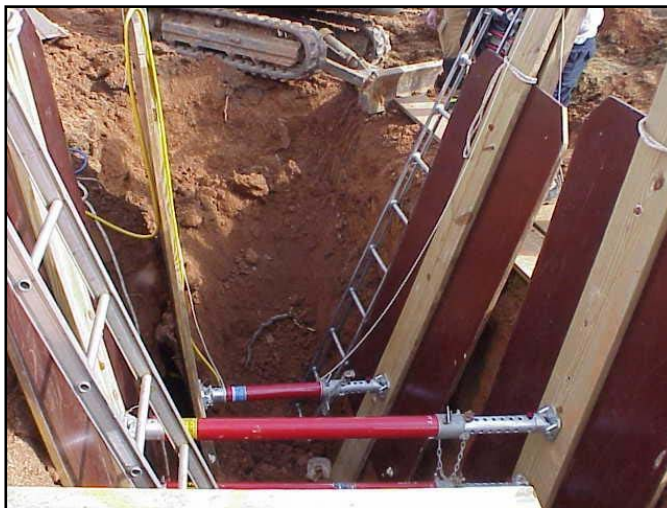
Photo 3. Illustrates the trench plates installed by the rescue squad. Photo courtesy of NCOSHA
