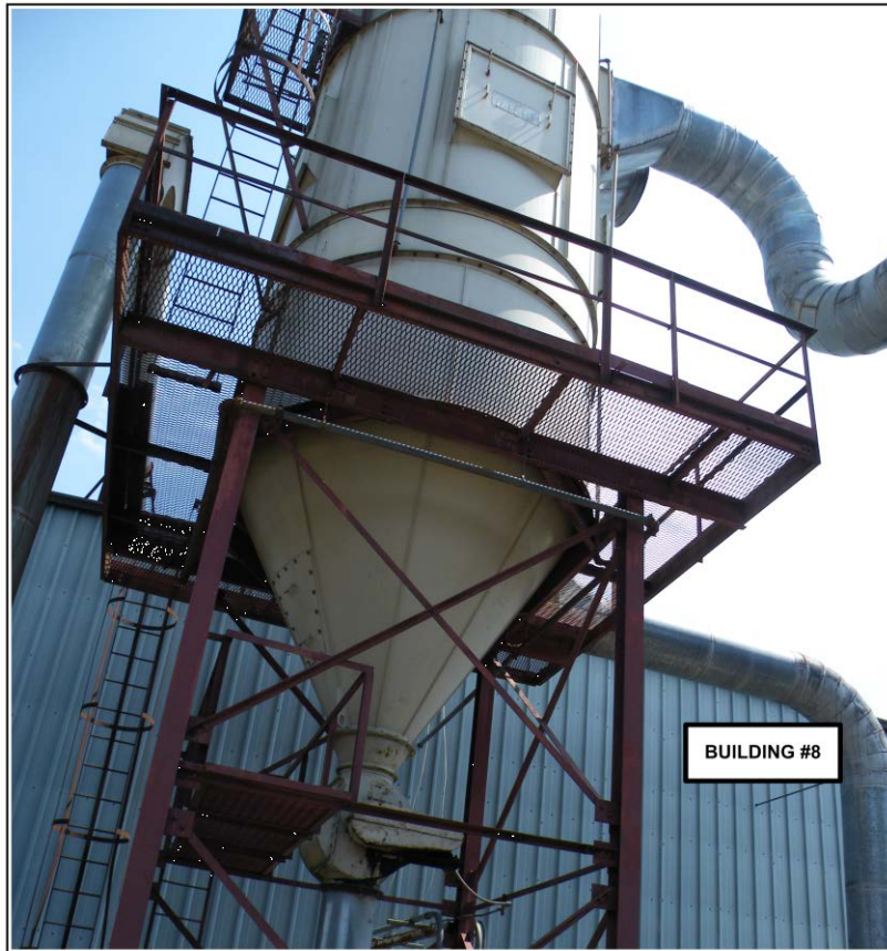
Photo 1. Dust collection unit. (Photo courtesy of NCDOL/OSH)
