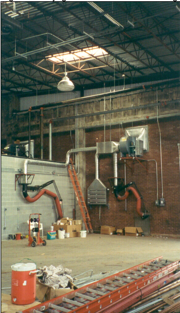
Figure 2. Skylight the decedent fell through
