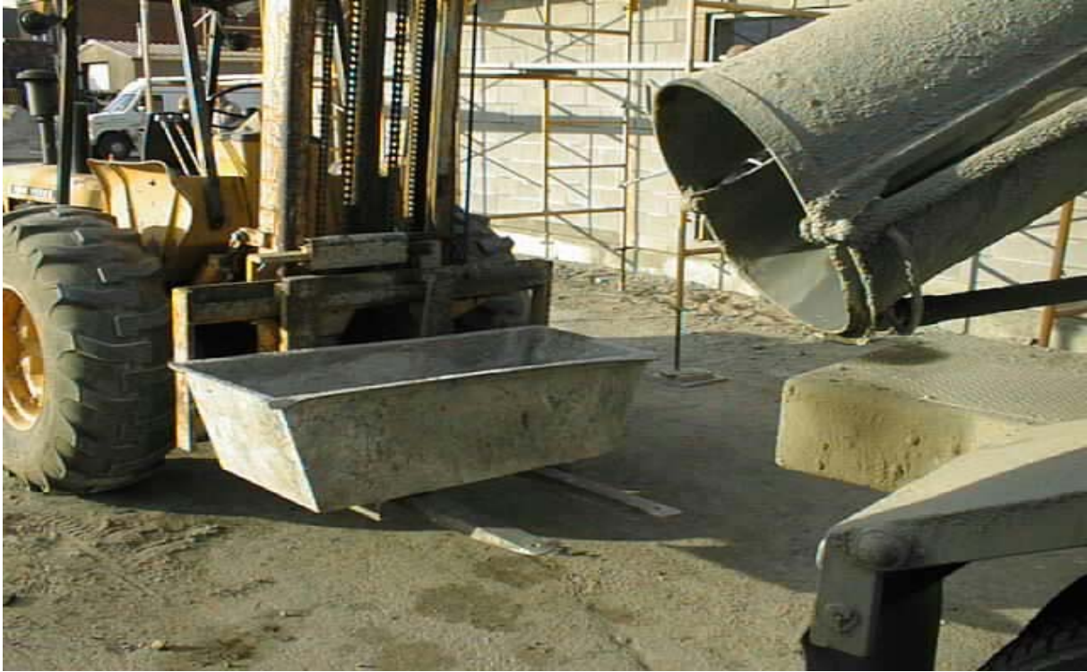
Picture # 6: Forklift and cement truck shortly after accident.
