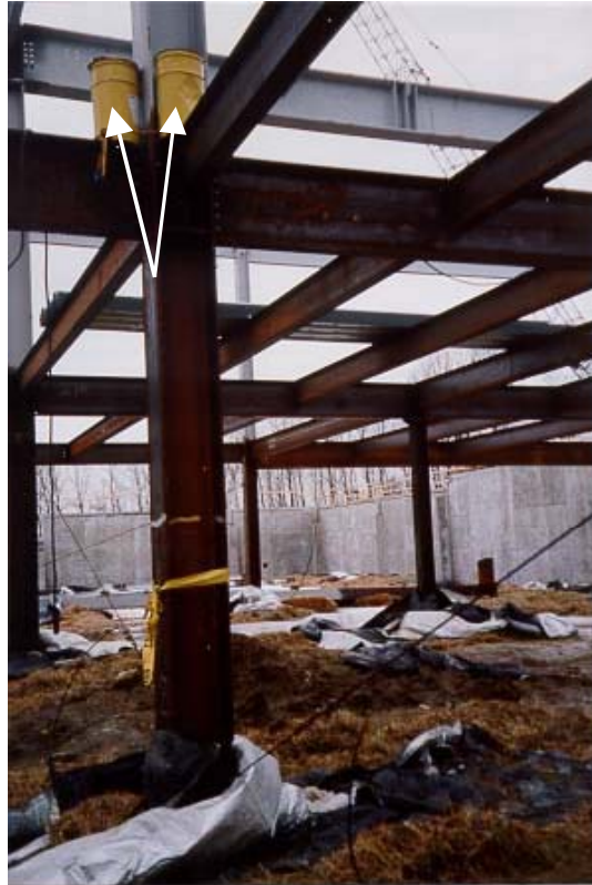
Figure 2 - Column with the two bolt kegs the victim was stepping around.
