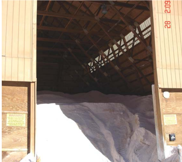
Photo 5. The entrance to the salt shed where the victim parked his truck at the time of the incident.
