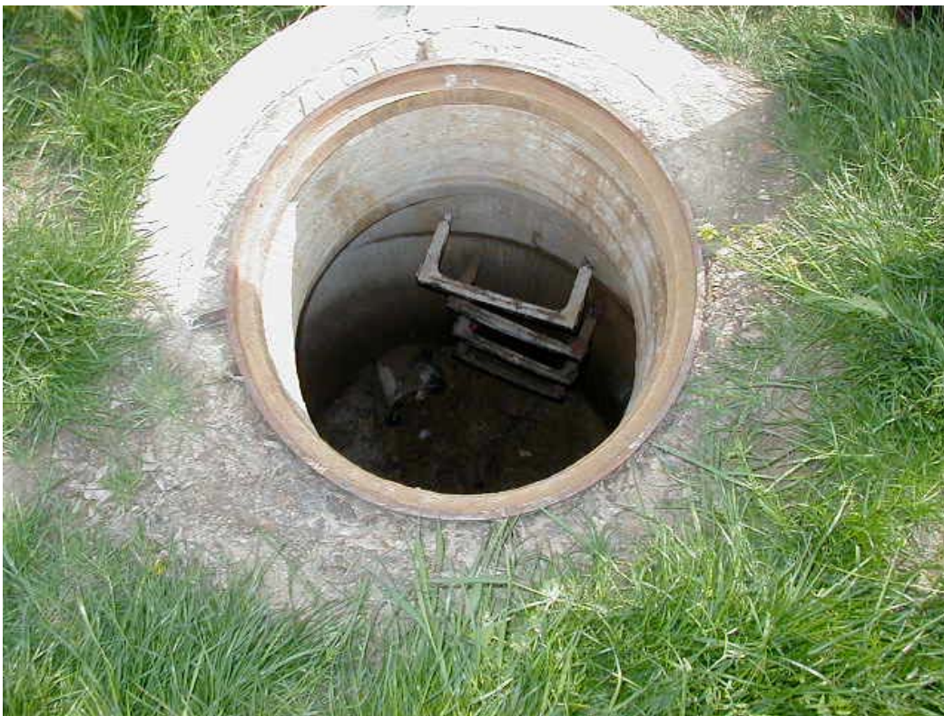
Figure 1. The landfill manhole where the fatality occurred.
