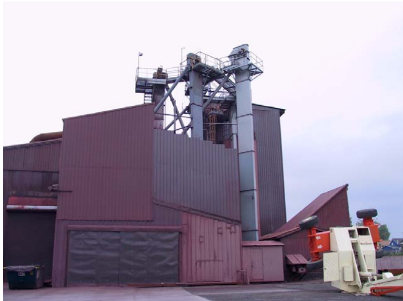
Figure 1. Bucket elevator that was being inspected by the victim during the fatal incident.
