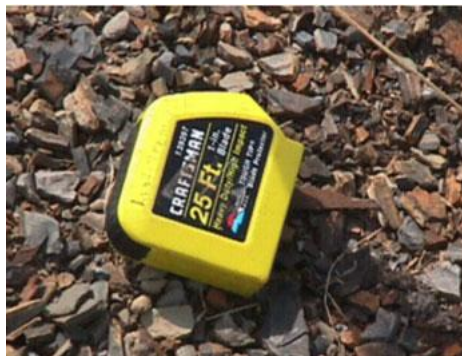
Figure 2. Photo shows the nature of the aggregate which was used to widen the road.
