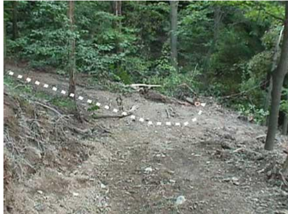
Figure 1. From left to right is the path the bulldozer followed while backing out of the newly constructed skid road. The end of the dotted line on the right depicts the nearly vertical drop-off.
