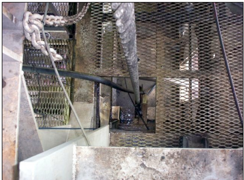
Figure 3. Unguarded floor opening where victim fell
