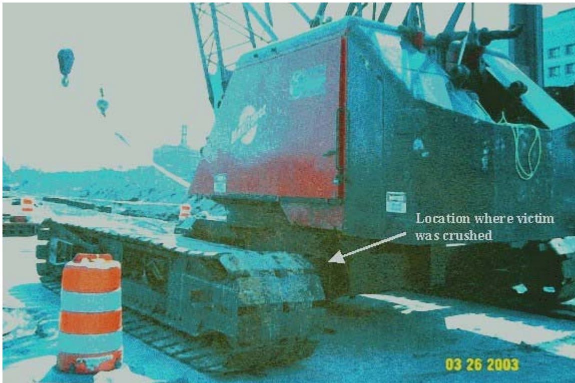
Figure 3 - Location where victim was crushed, between the left rear track and the superstructure.
