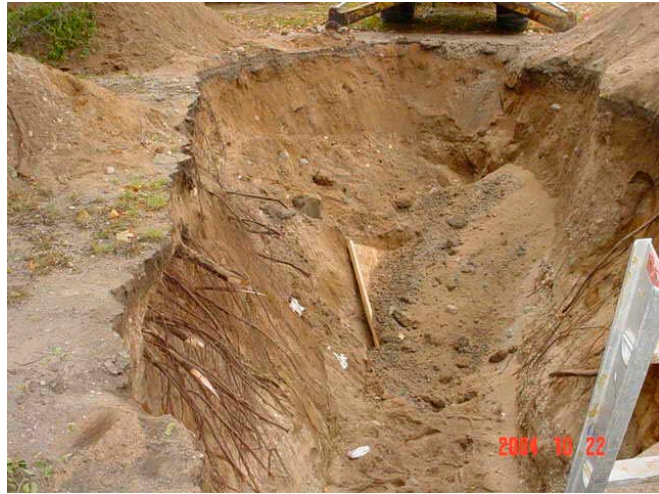
Figure 1. Picture of Trench after cave-in
