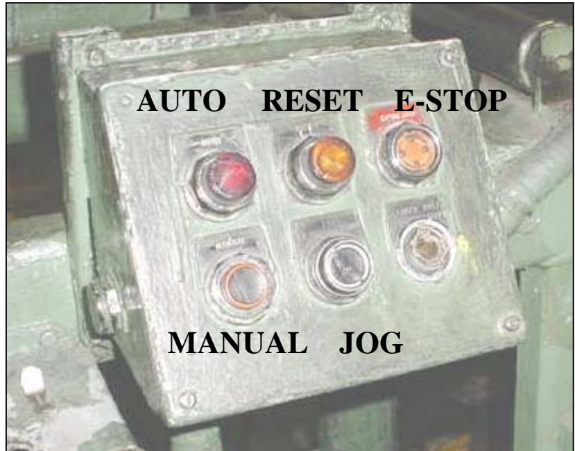
Figure 2. Control panel involved in the incident
