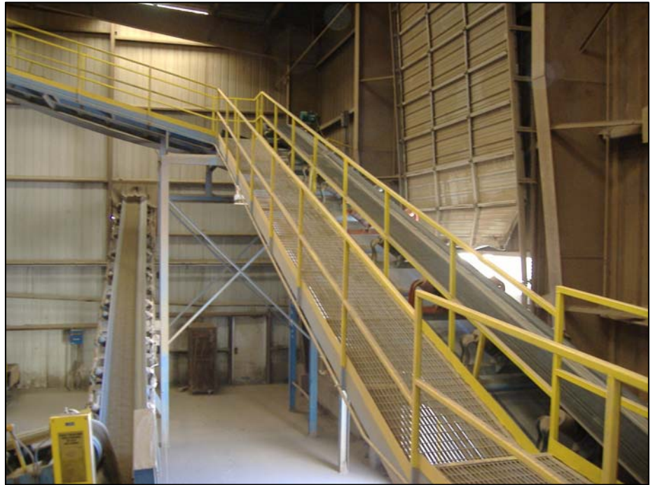
Figure 3. Catwalk system used to access the top of storage silos
