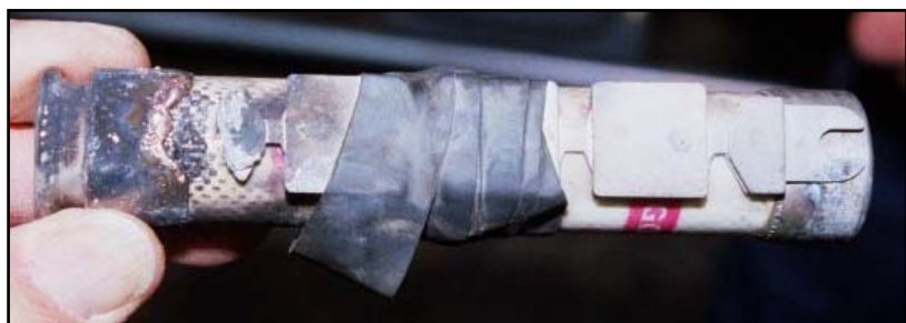
A melted fuse was repaired by taping a renewable fuse link on the outside.
