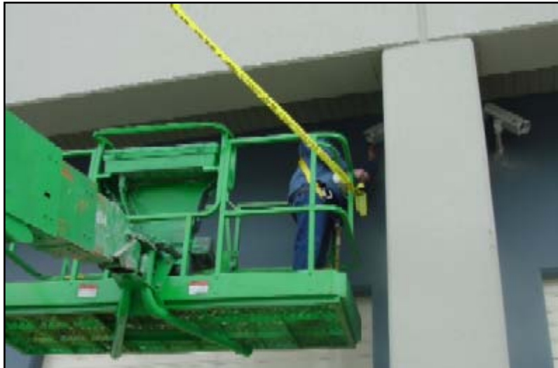
View of aerial platform during OR-OSHA investigation.
