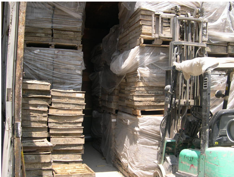
Exhibit 2. The incident scene showing the concrete and stone castings stacked on pallets in the curing oven. The pallets on the left collapsed onto the victim.
