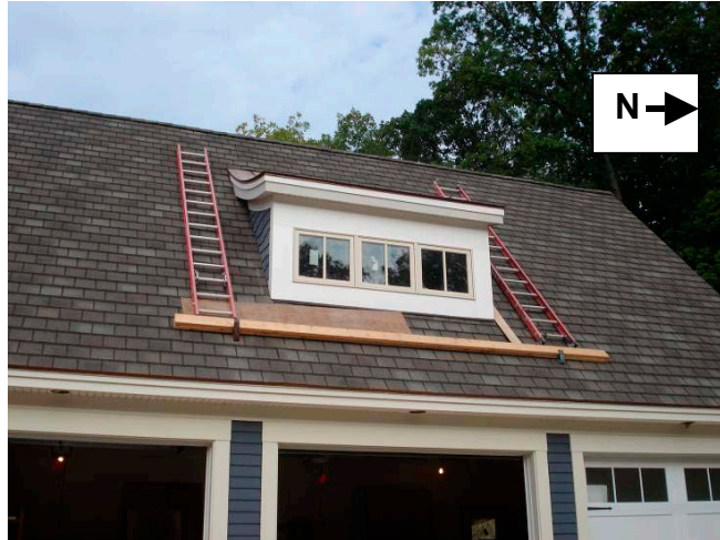
Figure 1. Re-enactment of incident scene showing placement of the roof brackets, planks and ladders.
