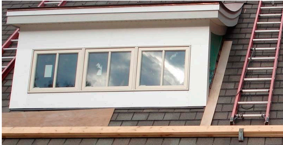
Figure 2. Another view of the re-enacted incident scene. Note placement of 2x6-inch planks
