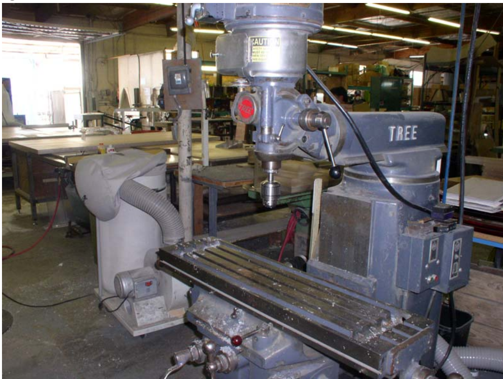
Exhibit 1. A picture of the vertical milling machine involved in the incident.
