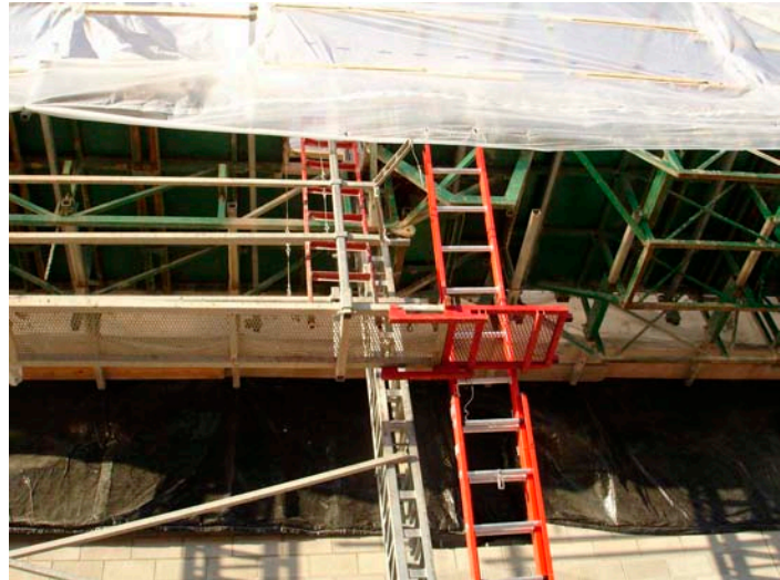
Figure 3. Extension ladder used to gain access to platform after the incident.
