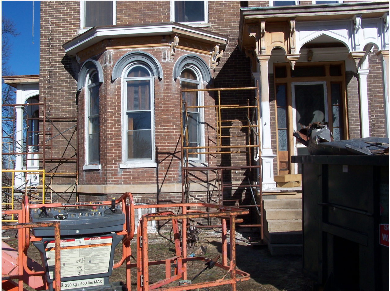
Alcove roofers were working on when foreman fell. Scaffolding was erected all around the alcove at the time of the incident.
