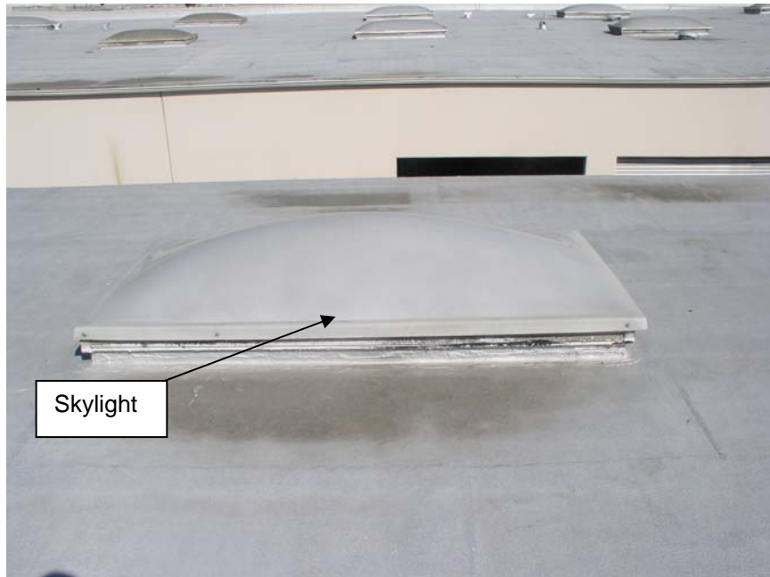
EXHIBIT 2. The skylight involved in the incident.
