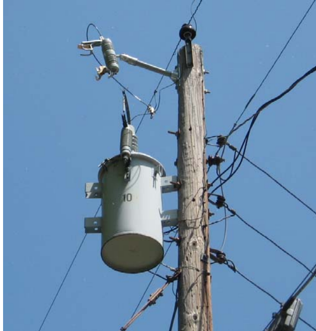
Figure 1. Transformer/can arrester involved in incident, looking north
