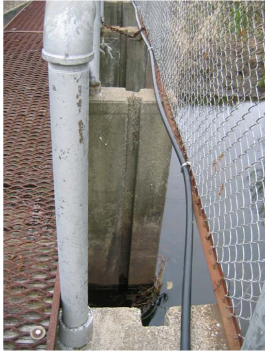
Figure 5. Channels holding stop logs
