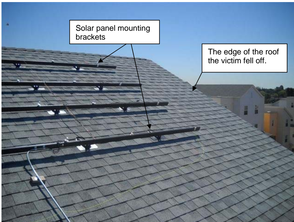
Exhibit 2. The mounting brackets for the solar panels and the roof's edge where the victim fell.
