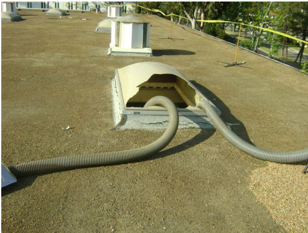
Exhibit 3. The skylight the victim fell through.
